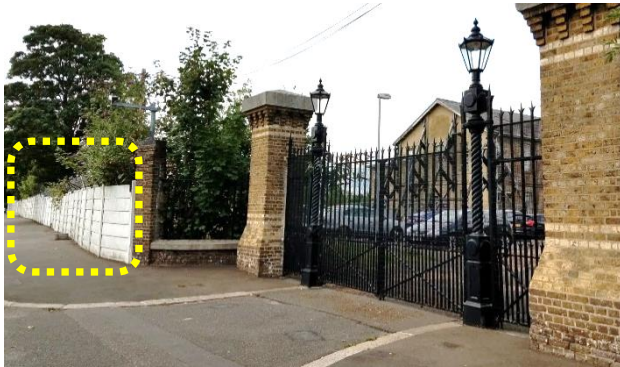
Figure 6.3.22a: Section of the wall can be removed (gate posts and gates must be kept)
