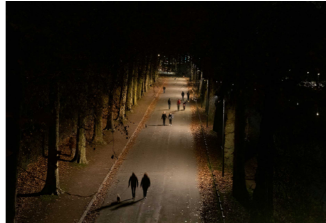
Fig A2.32 LED street lights in La Citadella, Lile. The lights are of different colour temperatures between 2,200K and 2,700K and also have motion detectors. They are programmed to adapt to the seasonal behaviour of bats © Schreder
