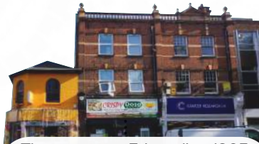
Three storeys Edwardian 1905 classic red brick with terracotta balustrade, keystones, and original pilasters
